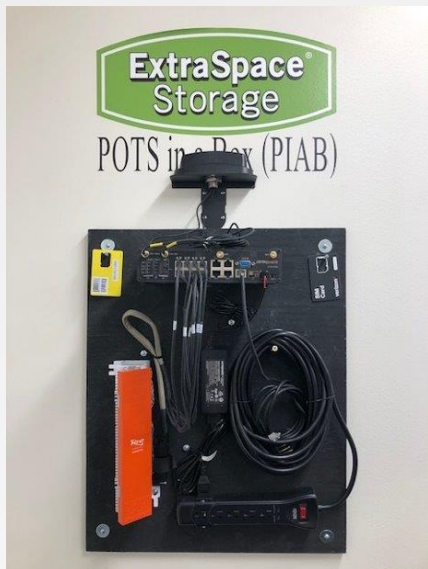
Dual SIM PIAB Copper replacement w/ 24-hour battery backup
