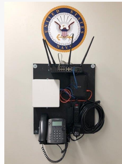
SD-WAN, w/ Broadband modem, LTE Backup, PIAB Copper replacement w/ 24-hour battery backup, Emergency Phone
